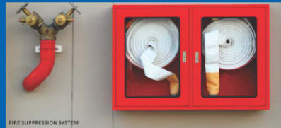
FIRE SUPPRESSION SYSTEM
