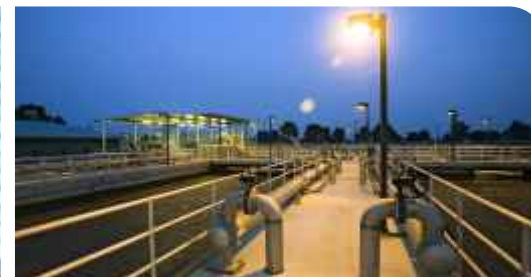
SEWERAGE TREATMENT PLANT
