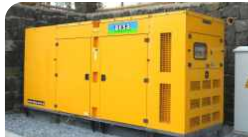
POWER BACKUP GENERATOR
