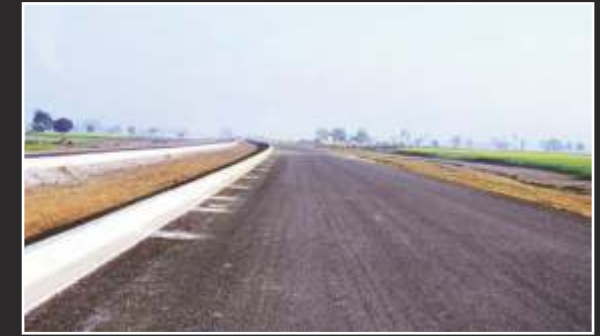
Actual photograph of the KMP expressway, nearing completion, close to the Raheja's Aranya City Site.
